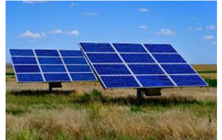
Solar Array (multiple panels)
